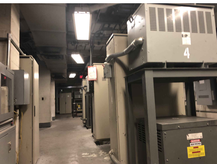
PHOTO 3 LIVE PANEL BOXES TO BE PROTECTED.
